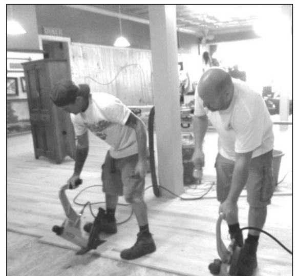
Volunteers select the correct size boards while Kris Sheffield and Larry Seville nail them to the underlayment.
